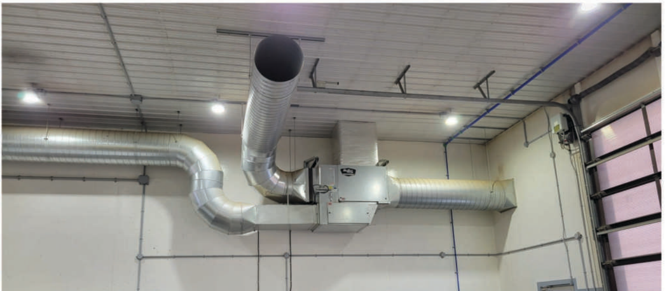
BA-HRV-50 Installed in a washbay
