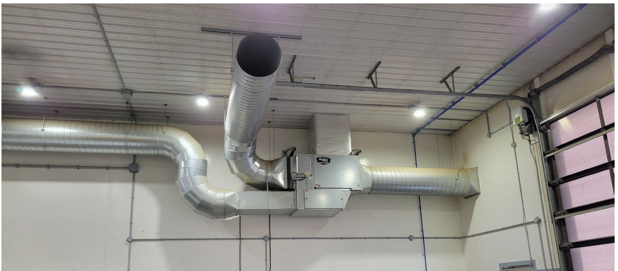
BA-HRV Installed in a washbay
